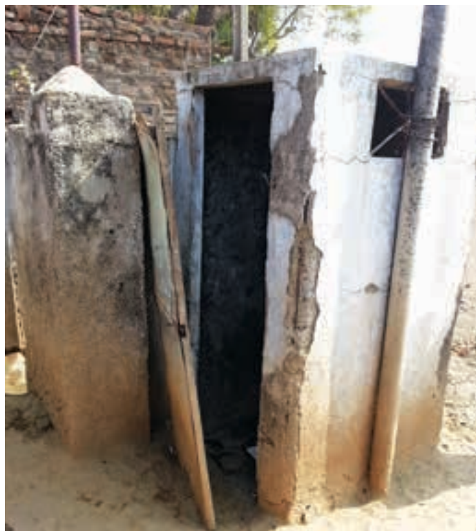
A toilet made from government funds under CRSP in Pimpalgaon. The toilet is dysfunctional currently
