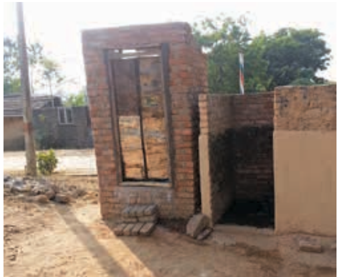
A toilet built under TSC still uses a make-shift gate and has no super-structure
